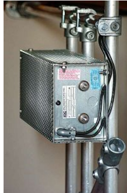
Figure 2.8: Electrical braking resistor for wind turbine.
