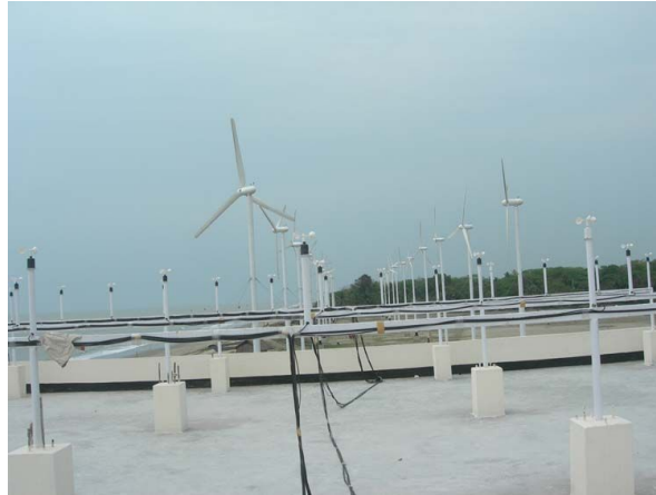
Figure 7.6: Anemometers and Wind Turbines of 1000 kWp Capacity Wind Battery Hybrid Power Project
