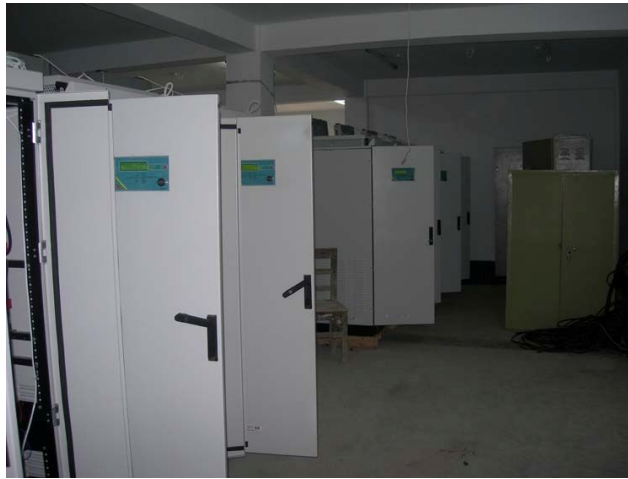
Figure 7.7: Control room of 1000 kWp Capacity Wind Battery Hybrid Power Project at Kutubdia Island
