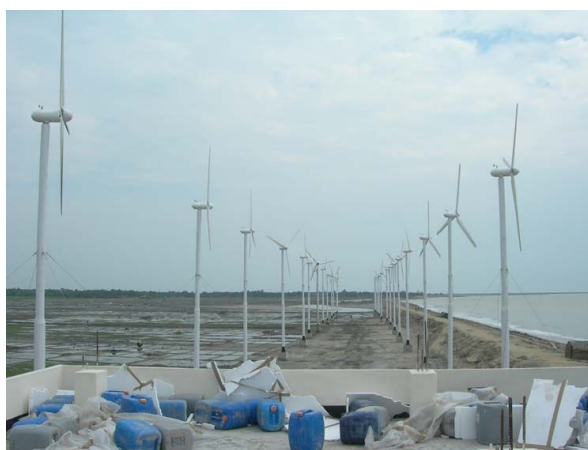
Figure 7.5: Wind Turbines of 1000 kWp Capacity Wind Battery Hybrid Power Project at Kutubdia Island
