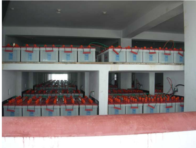
Figure 7.9: Battery Bank of 1000 kWp Capacity Wind Battery Hybrid Power Project at Kutubdia Island
