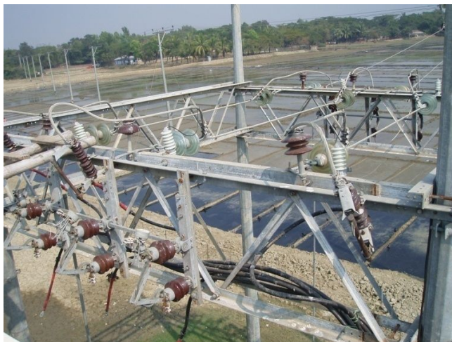
Figure 7.11: Overhead grid distribution line of 1000 kWp Capacity Wind Battery Hybrid Power Project 7.9.2 Grid Connected Wind Energy Project at Muhuri Dam areas by BPDB
