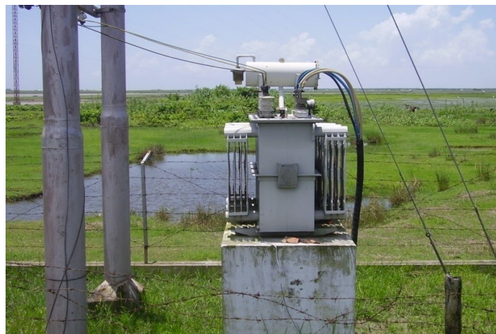
Figure 7.13: Step up transformer in Pilot project of 0.90 MW capacity of the Grid Connected Wind turbines in the Muhuri Dam areas at Feni District
