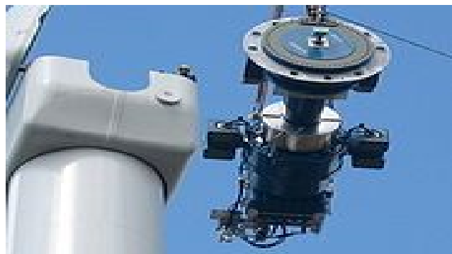
Figure 2.1: Components of a horizontal axis wind turbine (gearbox, rotor shaft and brake assembly) being lifted into position
