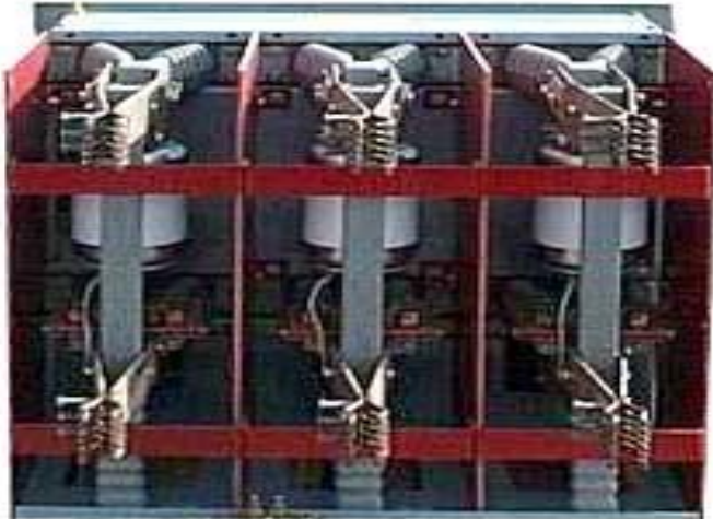
Fig: Vacuum circuit breaker, inside
