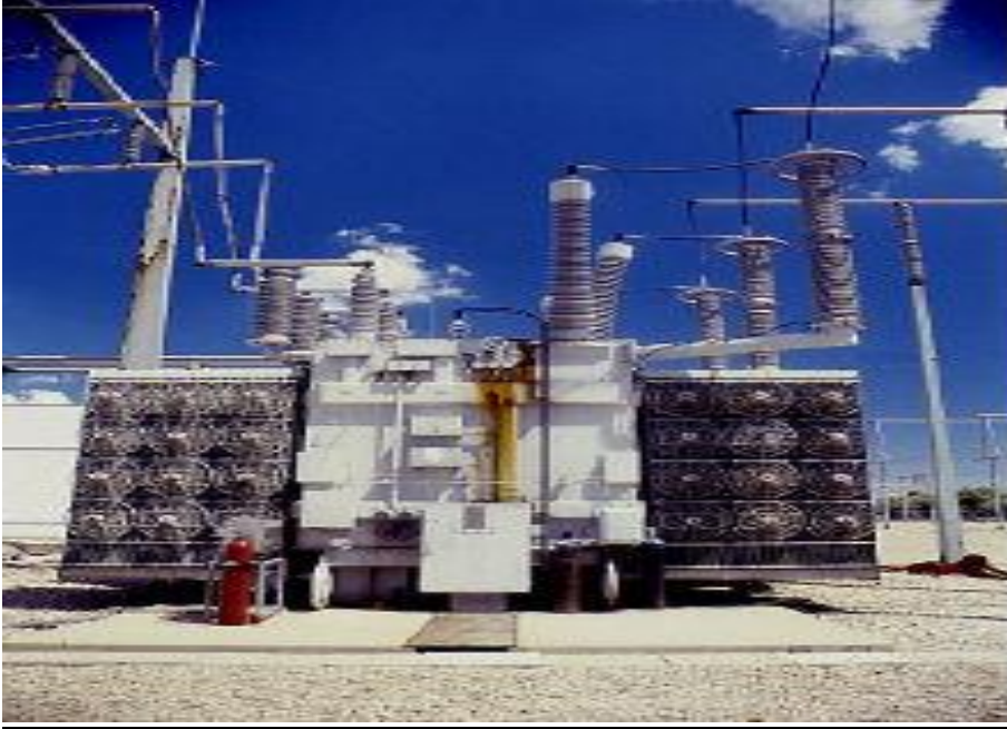
Fig: Power transformer, back view
