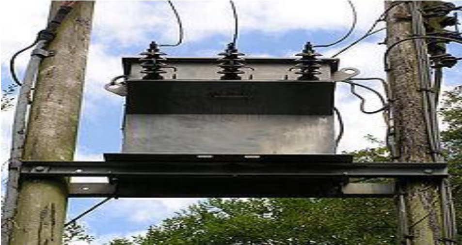
Fig: Three-phase step-down transformer mounted between two utility poles
