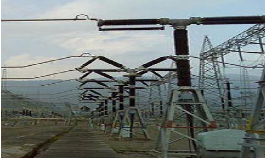
Fig: 400 kV SF 6 live tank circuit breakers
