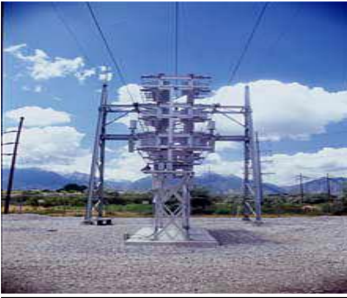
Fig: Capacitor bank, end view
