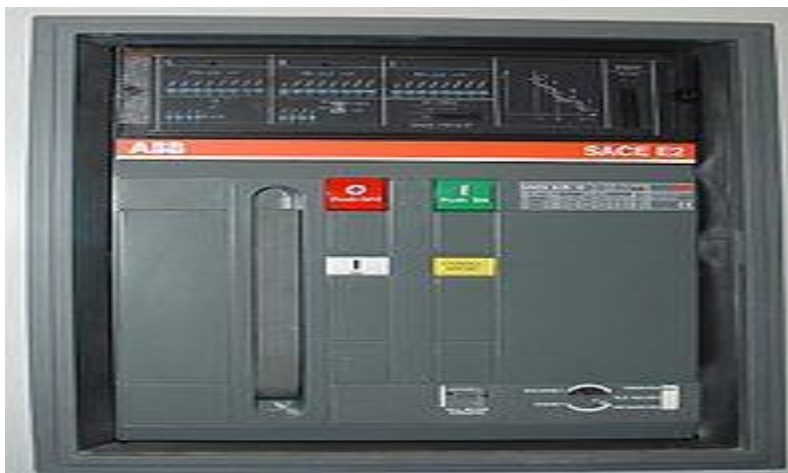
Fig: Front panel of a 1250 A air circuit breaker
