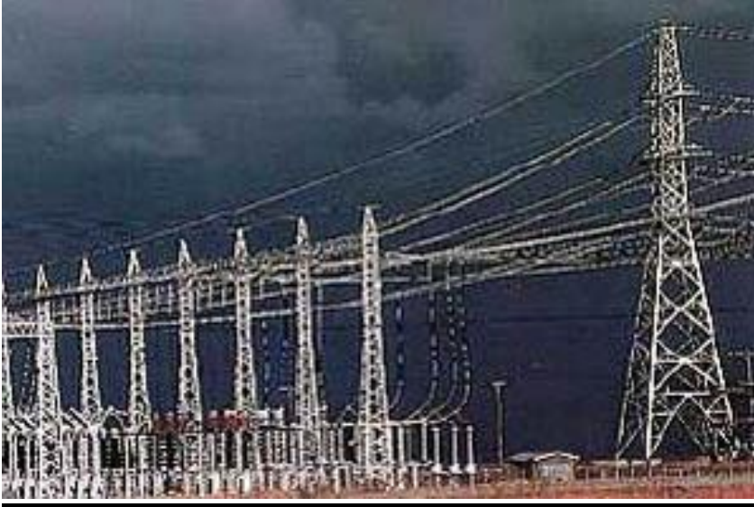
Fig: Step-up transmission substation to AC transmission lines
