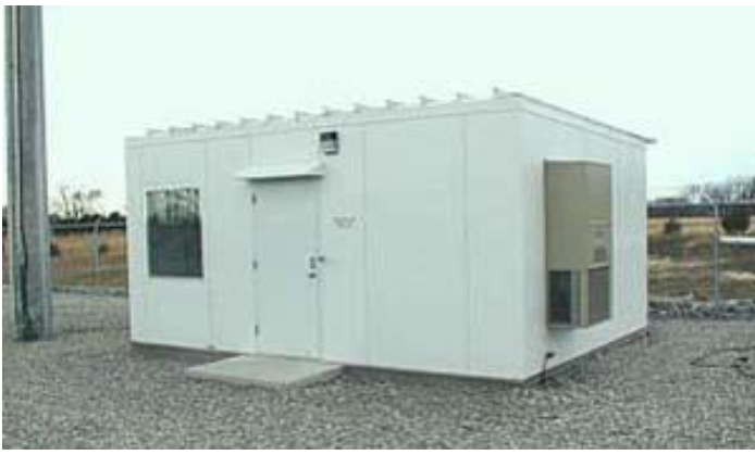
Fig: Substation control house
