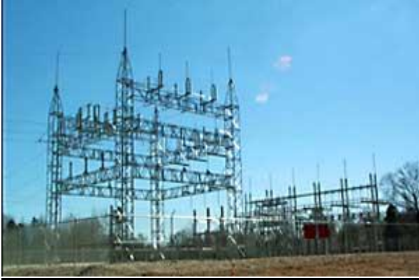
Fig: Distribution substation
