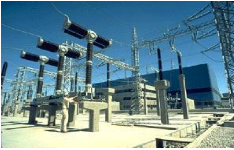
Fig: Step-up AC transmission substation
