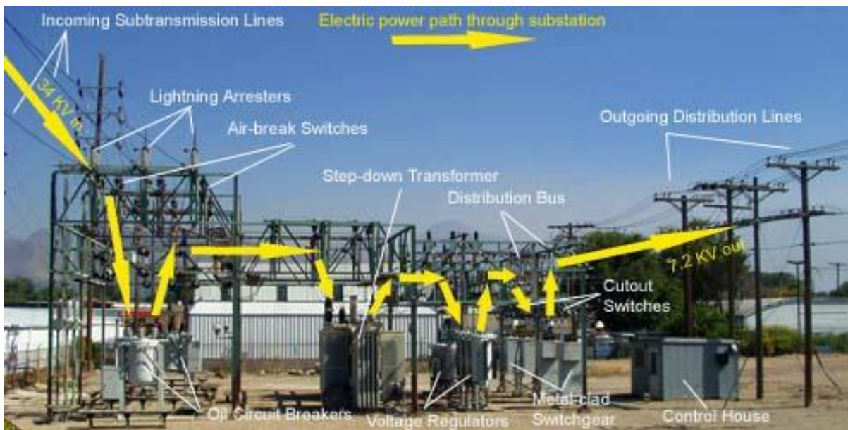
Fig: Electrical Substation
