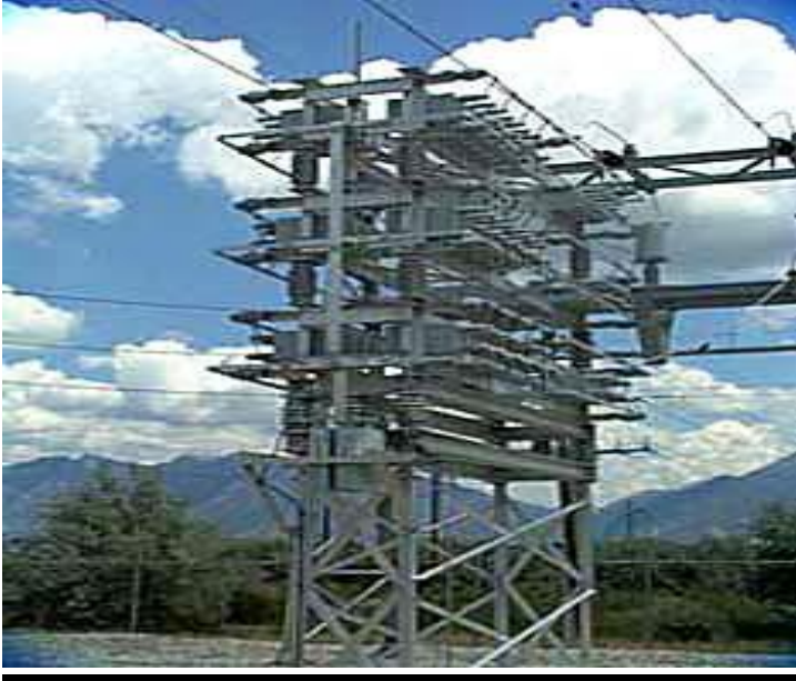
Fig: Capacitor bank, side view
