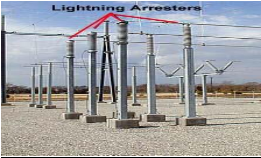
Fig. Lightning arresters on bus structures
