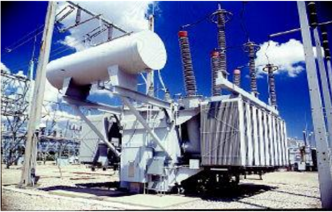
Fig: Power Transformer, front view
