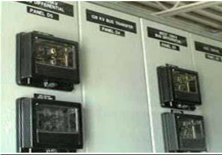
Fig: Substation control panel relay
