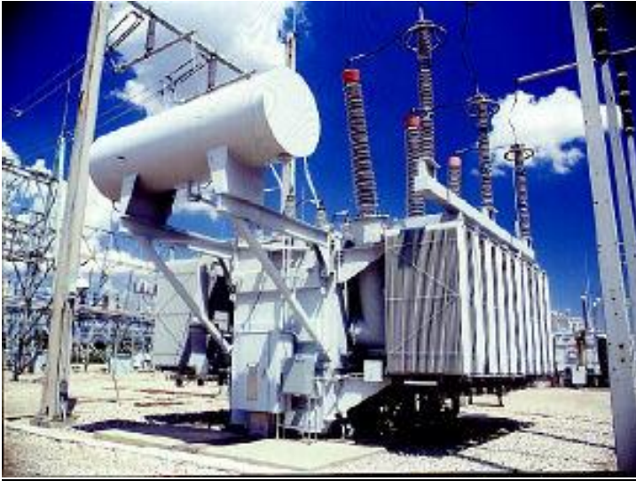
Fig: Step-down power transformer
