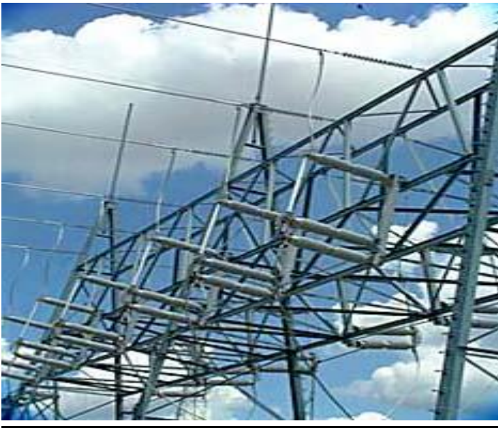
Fig: Circuit switchers
