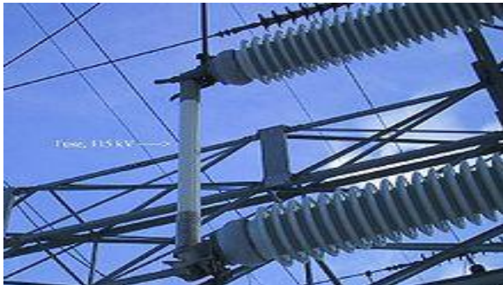
Fig: A set of pole-top fusible cutouts with one fuse blown, protecting a transformer- the white tube on the left is hanging down
