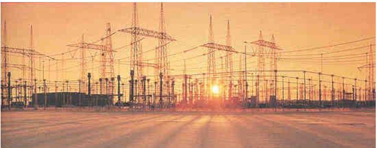
Fig: Step-down transmission substation
