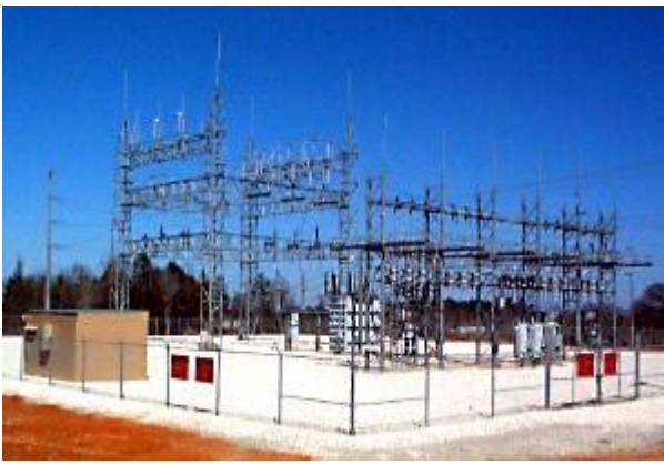
Fig: Distribution substation
