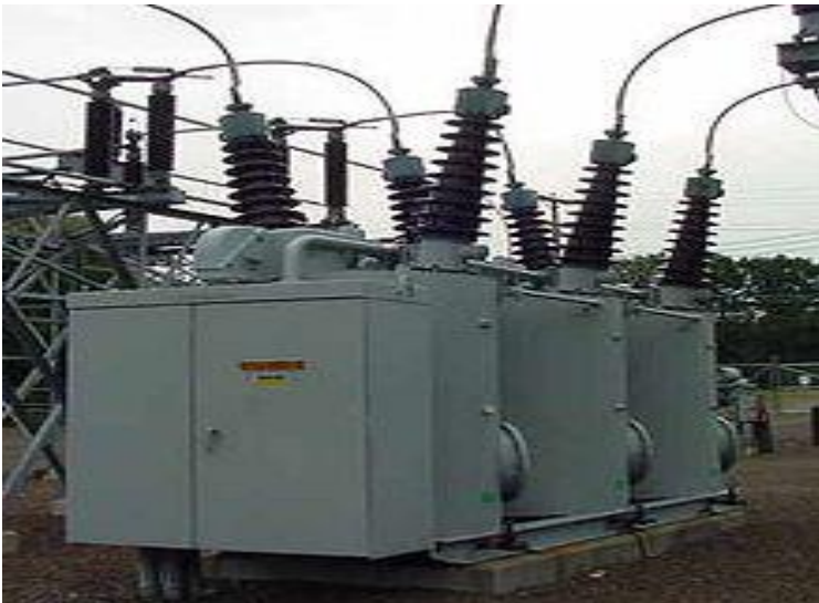
Fig: 115 kV bulk oil circuit breaker
