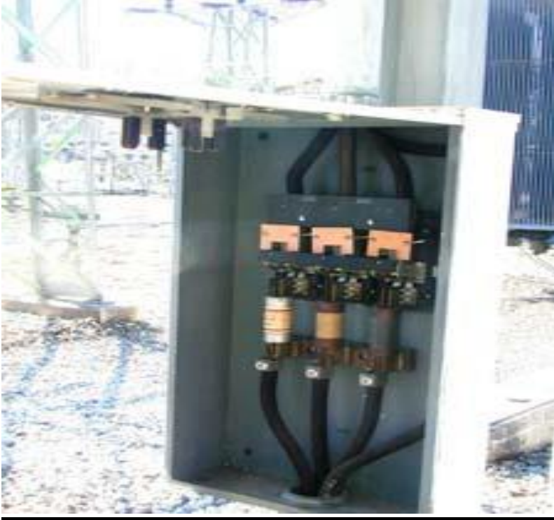
Fig: High voltage fuses in a switch box
