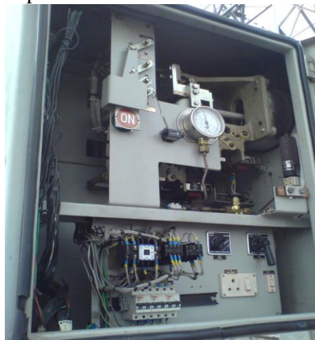
Figure: A installed SF 6 Circuit Breaker
