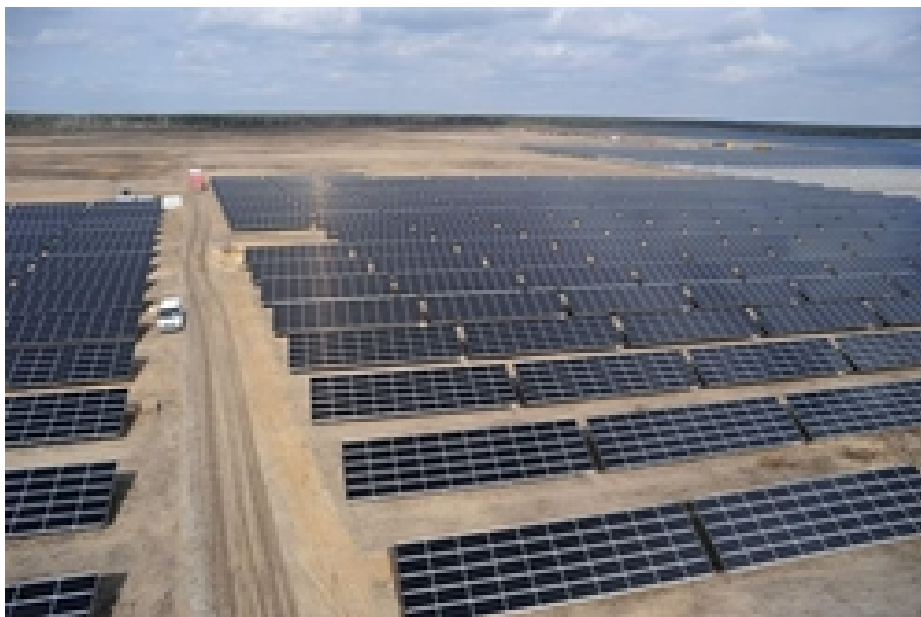
World largest solar park (Spain)
