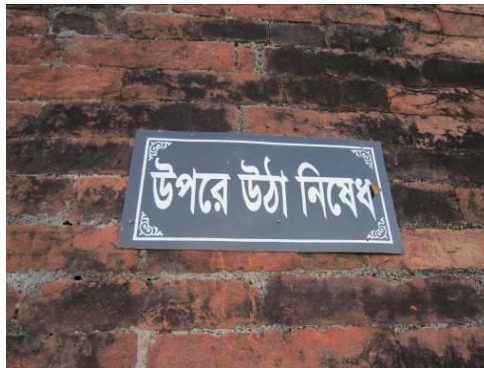
Figure 4: Restriction notice is attached on the Cell Wall by using nail and that is harmful for the brick by itself (Source: Authors)
