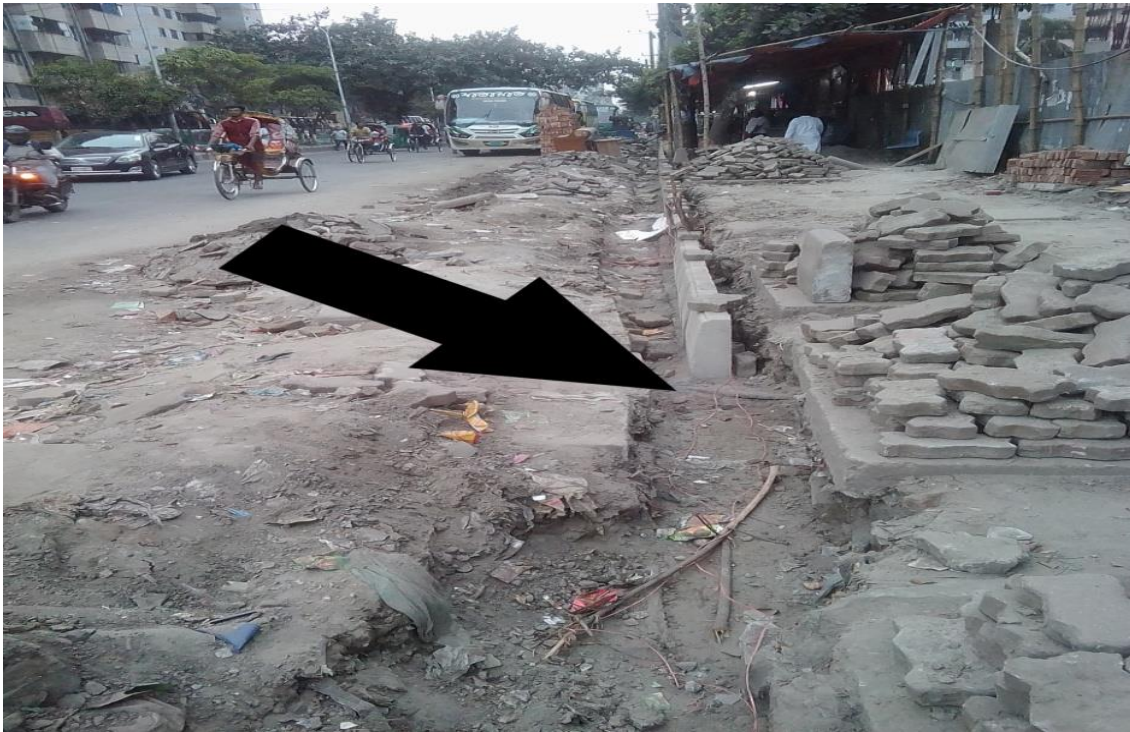
Photo 4.22: Road Side Damage
