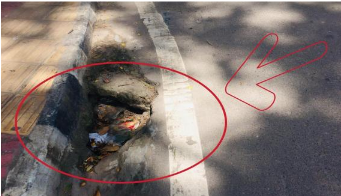
Photo 4.5: Poor drainage surface with waste of Tigerpass intersection
