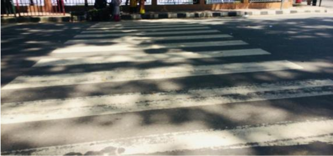
Photo 4.6: Poor zebra crossing marking quality of Tigerpass intersection.
