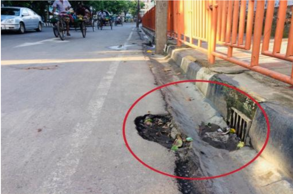
Photo 4.2: Damage road surface of Tigerpass intersection
