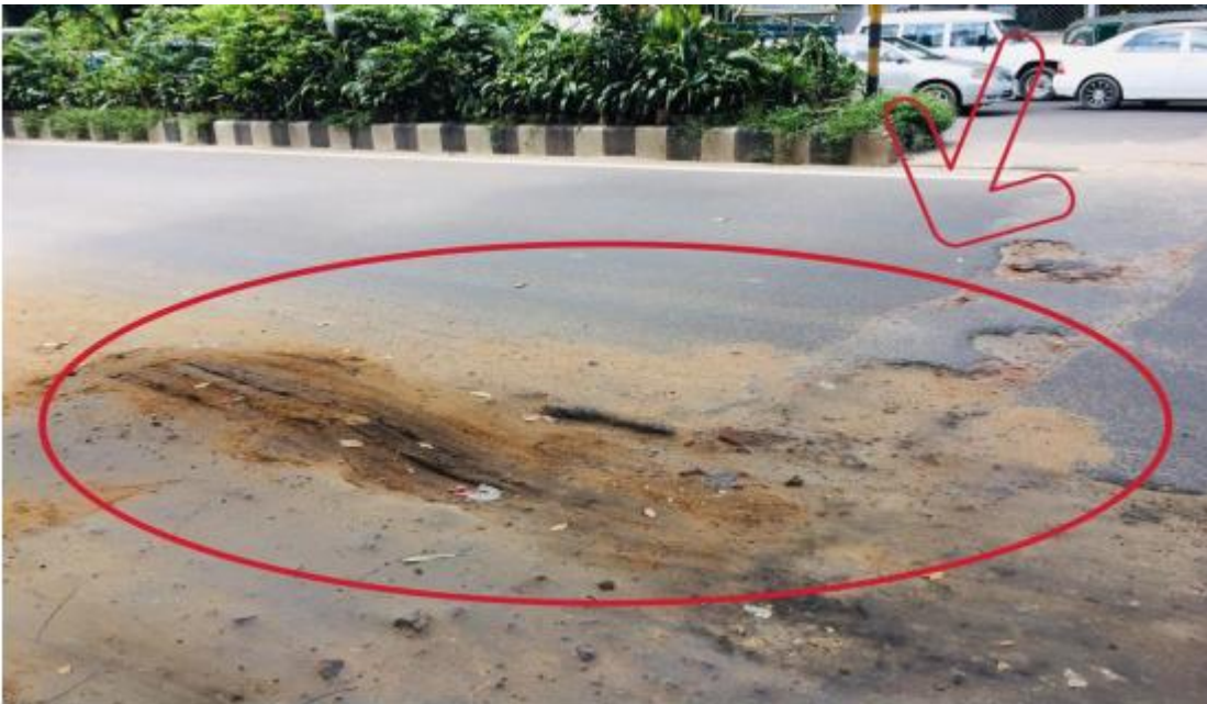
Photo 4.1: Poor surface quality of Tigerpass intersection.
