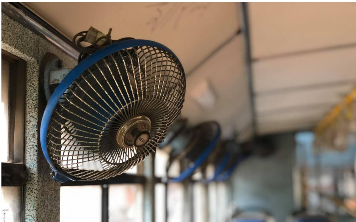
Photo 4.10: BRTC Bus (Fan Facilities)
