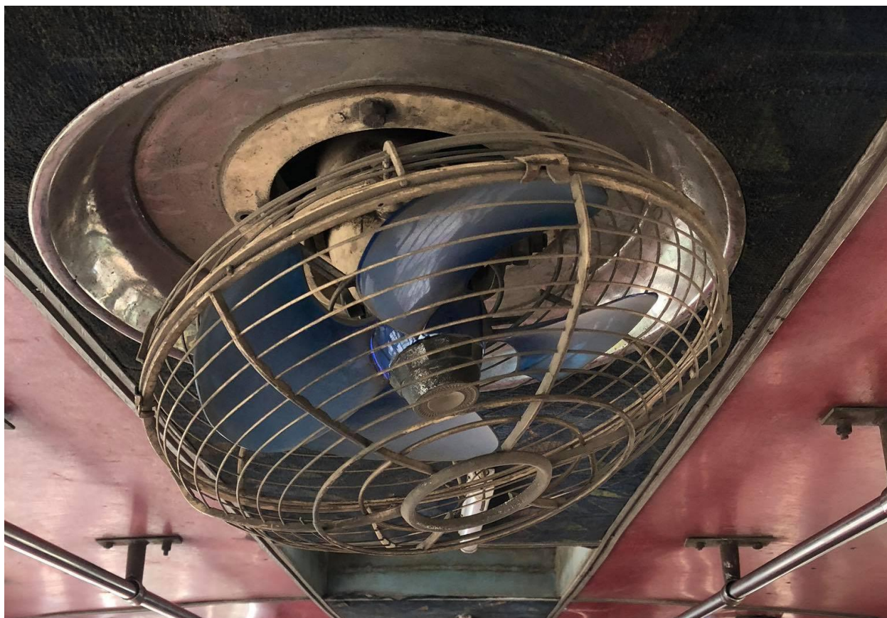
Photo 4.21: Local Bus (Fan Facilities)
