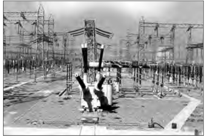
FIGURE 24.6 Spare converter transformer in the switchyard of an HVDC station.
