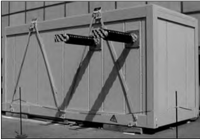
FIGURE 24.27 Compact outdoor container with an active dc filter.
