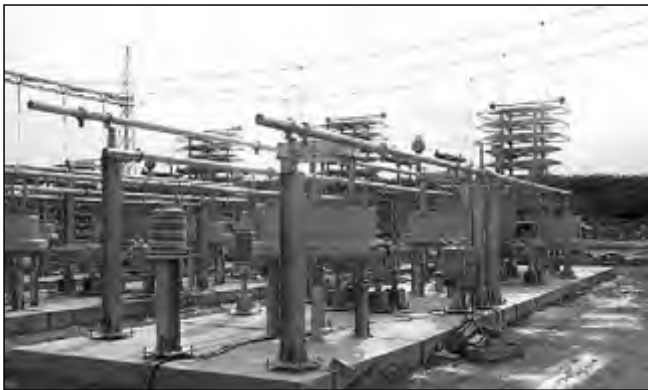
FIGURE 24.28 Installation of triple-tuned filter at the Gurun Station in Malaysia.
