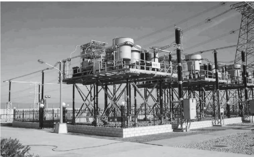
Fig. 1.15. Series Compensation (Series Capacitor) (Source: ABB)
